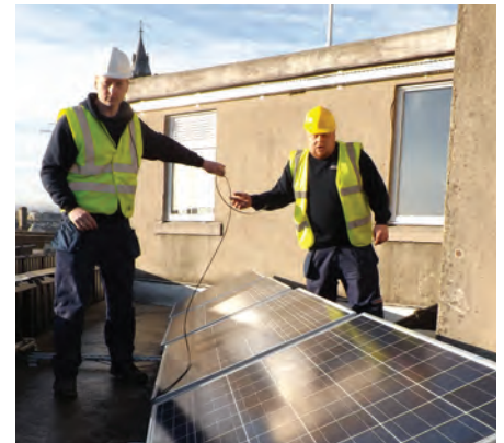
Rooftop solar panels
